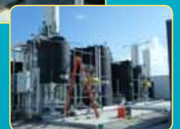
MBR Pilot System—Overview of Anoxic and Aeration Tanks
