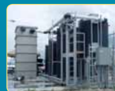
MBR Membrane Tank (Stainless Steel)
