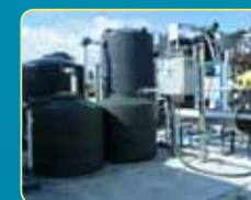
Advanced Oxidation Process Finish Water Stabilization Tanks
