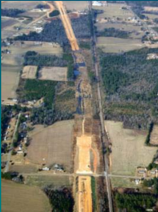
Wetland Loss to Highway Construction
